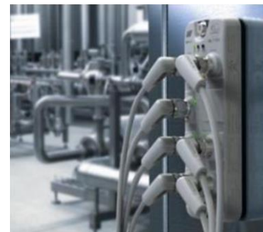
Fig. 1. Example of a 1st gen. 1 IO-Link Box
