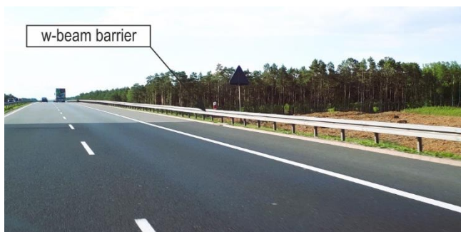
Fig. 1. Example of a w-beam barrier.
